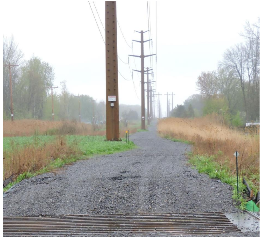
Example of double circuit structure
