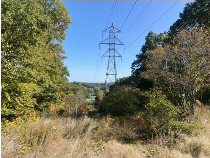
Typical E5/F6 lattice tower structure
